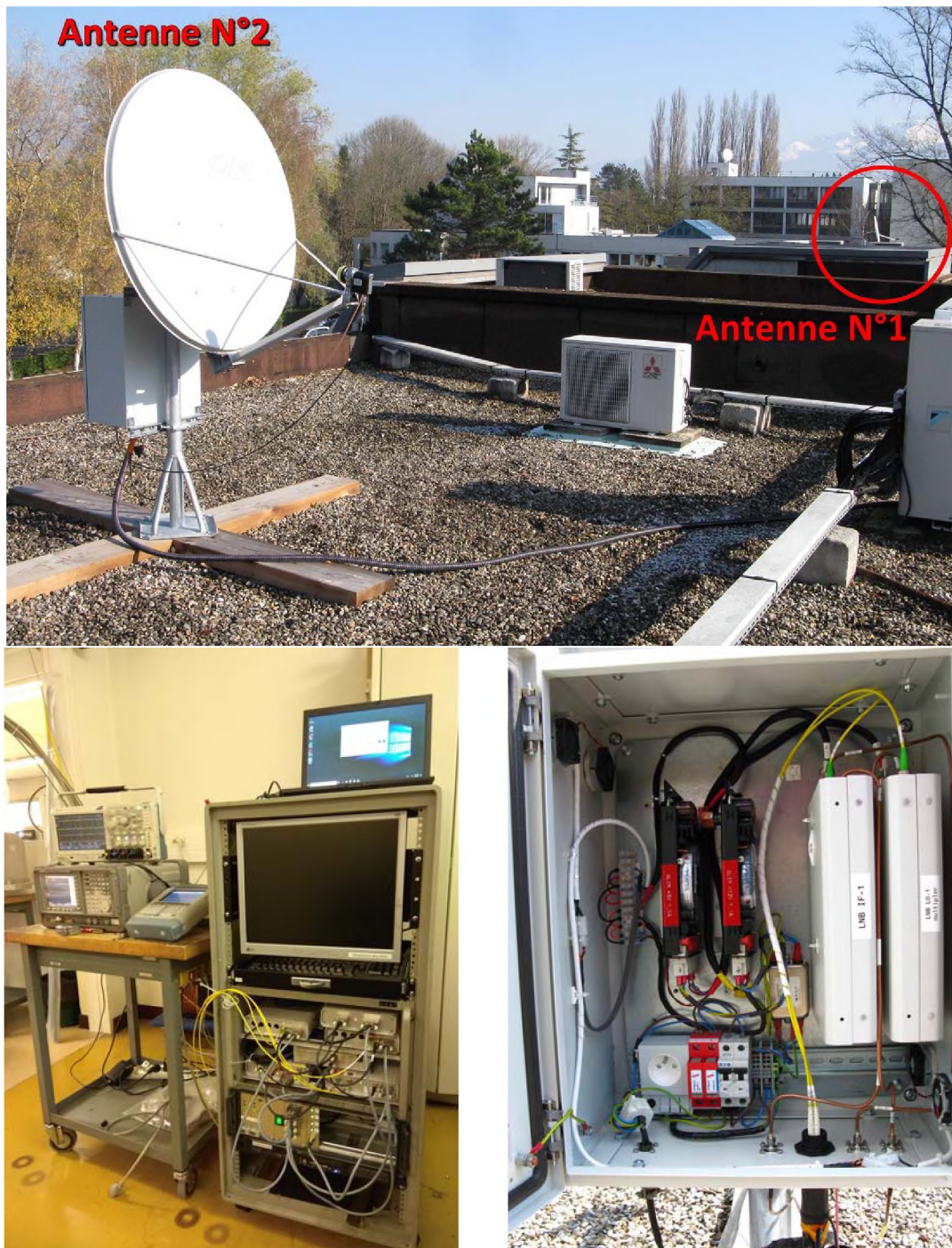
Figure 4: Top: Antennas on the IRAM headquarters roof in Grenoble. Bottom left) Indoor rack of electronics and control pc, Bottom right) Outdoor rack of electronics.
